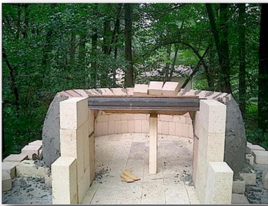
8.1. An angle iron framed opening. Note the lack of a reveal for the door jam (don't do this).
