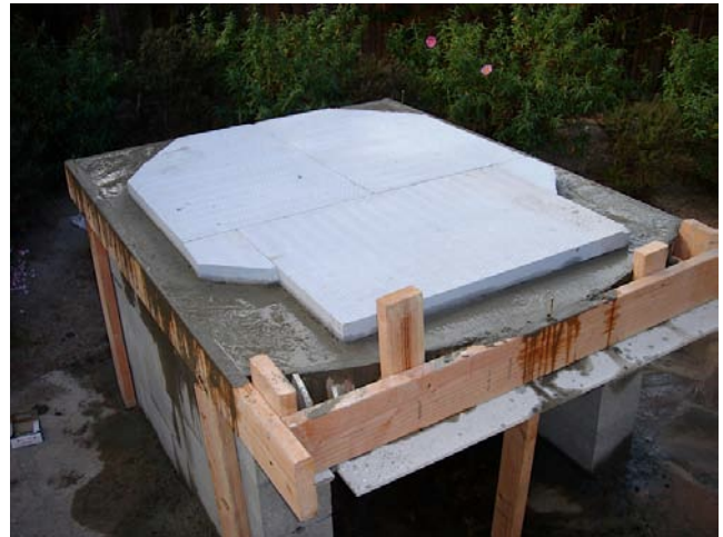
4.2. FB Board on damp concrete.
